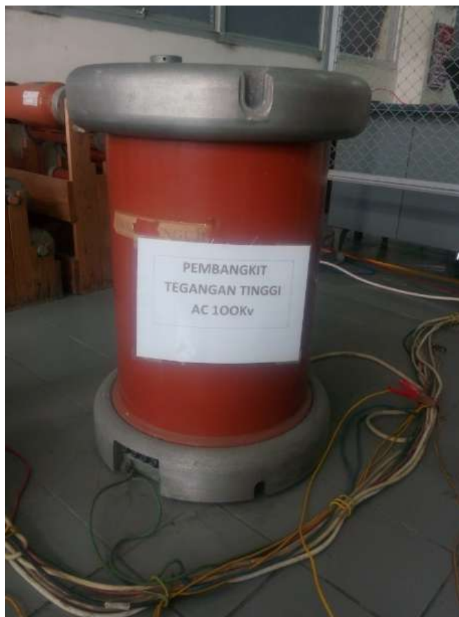
Trafo Step up “ Cascade Connection ”
